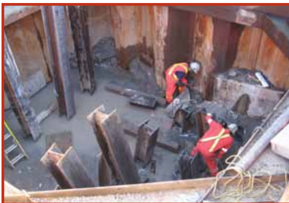
Heavy Civil, Water Cut-Off, Orangeville, Ontario A combination of cement grout and chemical grout is used to cut off large flows of soil and water in bridge construction.
