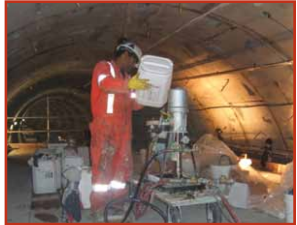
Tunnel Construction, Chemical Grouting, Edmonton, Alberta Chemical grout is used to stabilize soil, cut off active water flow and seal leaking joints in various forms of tunnel construction.
