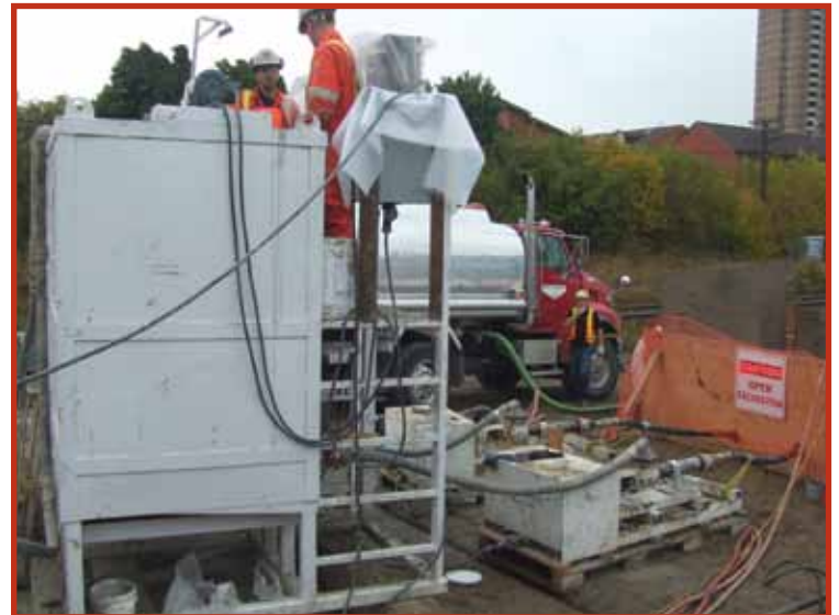
Utility Services, Cellular Grouting, Toronto, Ontario Light weight cellular grout is used to backfill casings after delicate conduits and high voltage cables are installed beneath railroad tracks, airport runways or roadways.
