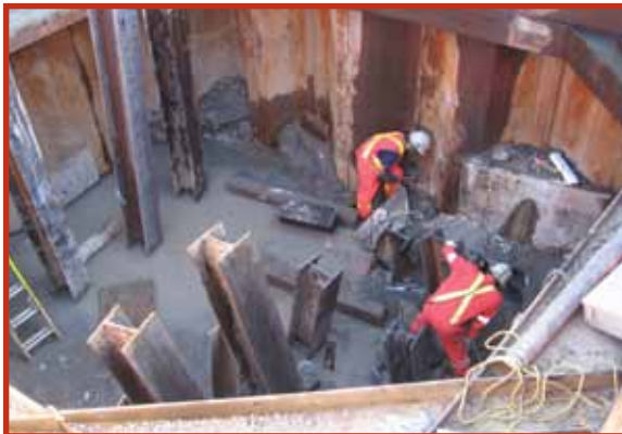
Heavy Civil, Water Cut-Off, Orangeville, Ontario A combination of cement grout and chemical grout is used to cut off large flow of soil and water in bridge construction.
